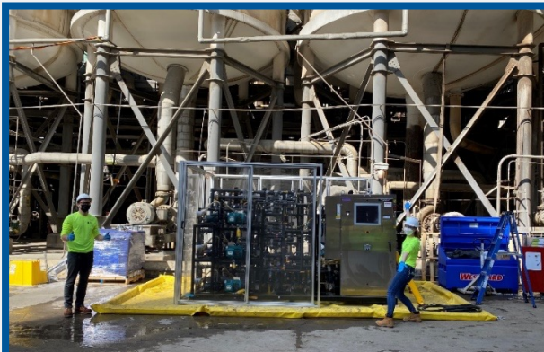
Via Separations' pilot system installed for the first time at a customer's location.
