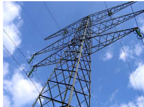
TCIP researchers work to provide end-to-end secure and real-time power grid monitoring and control. Credit: http://commons.wikimedia.org/wiki/File:Ligne_haute-tension.jpg .
