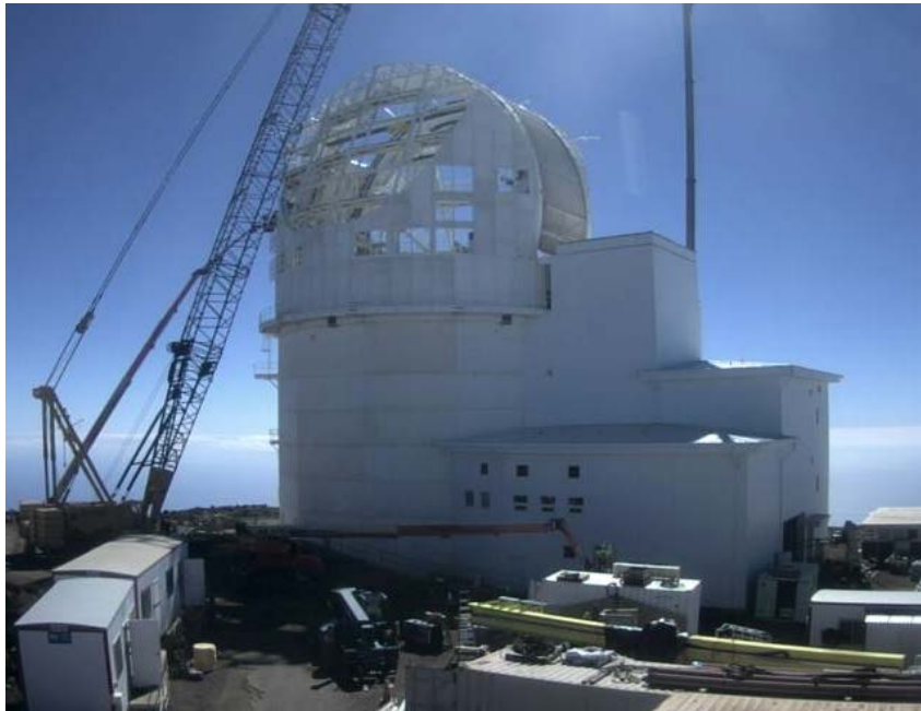
Telescope enclosure assembly underway at the DKIST site on Haleakala, Maui, HI, November 2015. Credit: DKIST project web camera.
