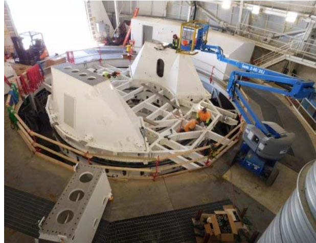
Installation of the saddle sections of the DKIST telescope mount assembly (TMA), March 2017. Credit: P. Jeffers, DKIST.
