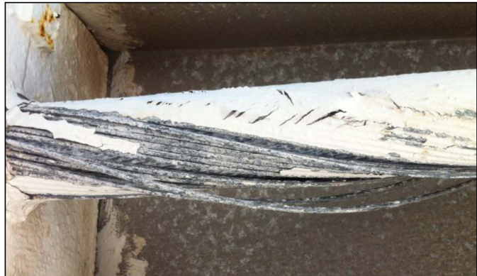
Figure 21: Multiple wire breaks observed at splice near tower end of cable M8-4 on 1/14/2014 (photo: NAIC Arecibo Observatory, a facility of the NSF).
