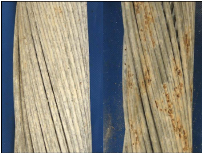
Figure 30: Oxidation of galvanizing zinc (left) and wire steel (right) in second wire layer of an original M4 cable (photos: Socotec).
