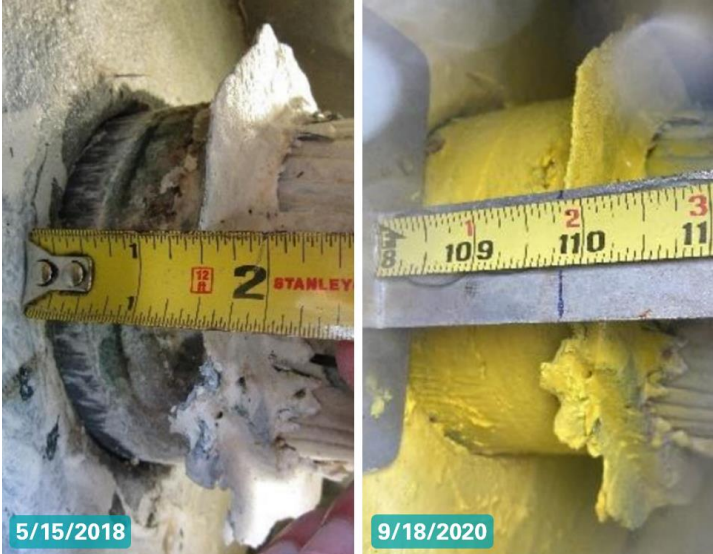
Figure 24: Cable slip increase measured at socket B12W_G (photos: NAIC Arecibo Observatory, a facility of the NSF).
