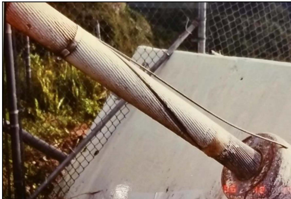
Figure 20: Single wire break observed at ground end of cable B4-1 on 12/12/1996 (photo: NAIC Arecibo Observatory, a facility of the NSF).
