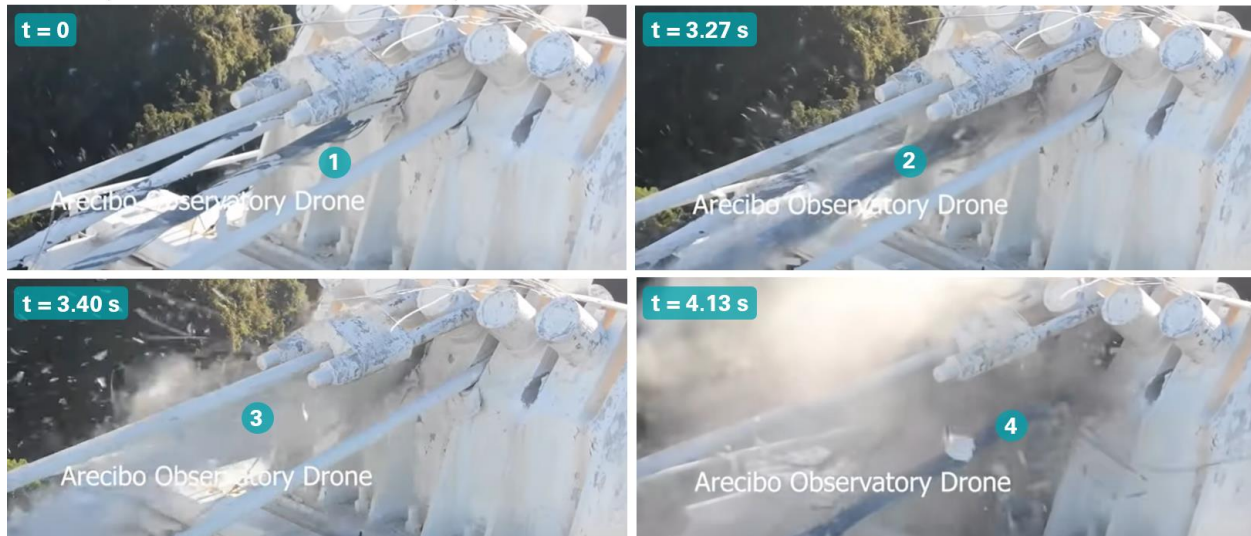
Figure 29: Progressive failure of original main cables at top of Tower 4. (still images of drone video by NAIC Arecibo Observatory, a facility of the NSF. Intermediate still images are provided in Appendix E.)
