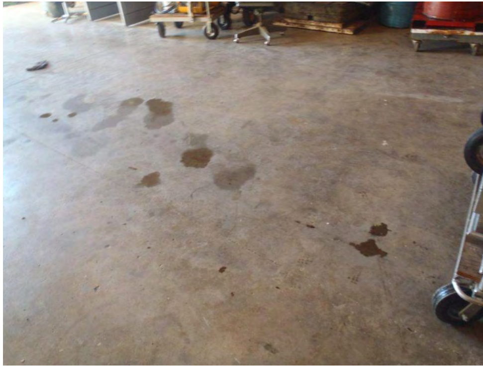
Photo 97: Staining of concrete floor inside GBT warehouse.
