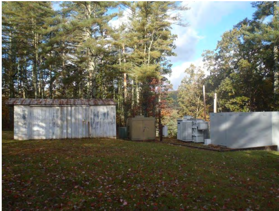
Photo 78: Electrical substation facing north.
