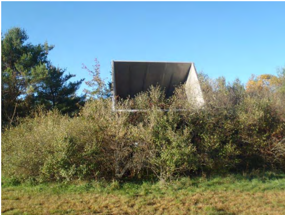
Photo 70: Top of Little Big Horn antenna facing southwest.
