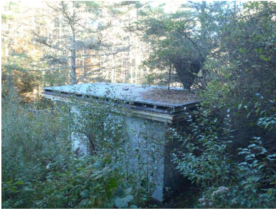
Photo 71: Base of Little Big Horn antenna facing north.
