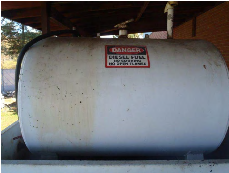
Photo 98: Diesel fuel AST behind Warehouse.
