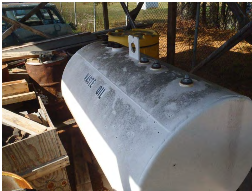
Photo 100: Waste oil AST at Work Area outside storage yard.
