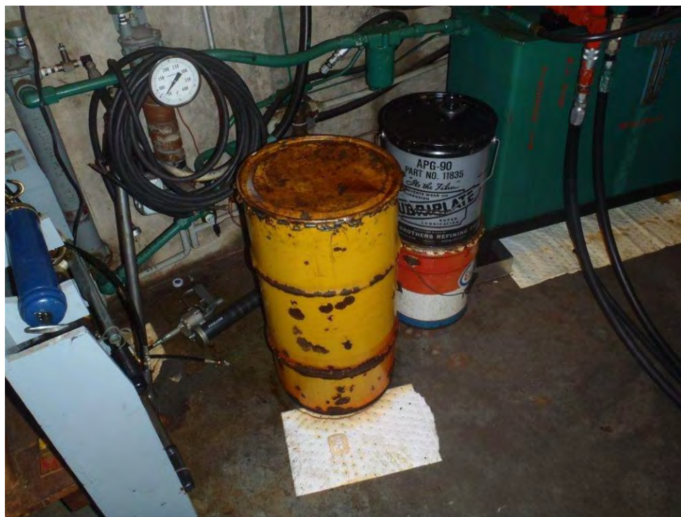
Photo 96: Drum leak at 43-meter Telescope.
