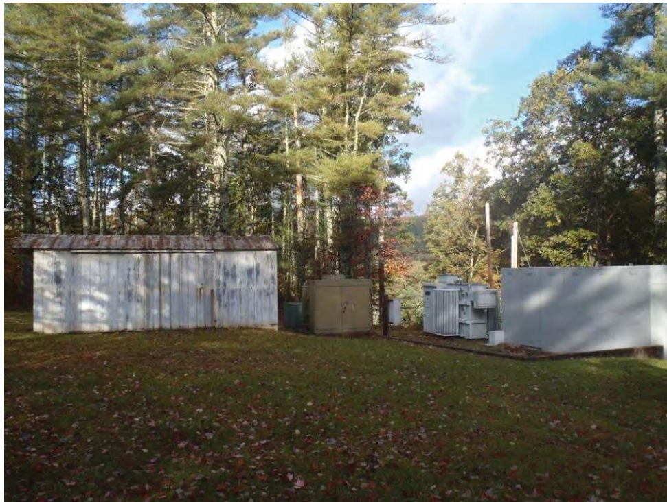
Photo 78: Electrical substation facing north.
