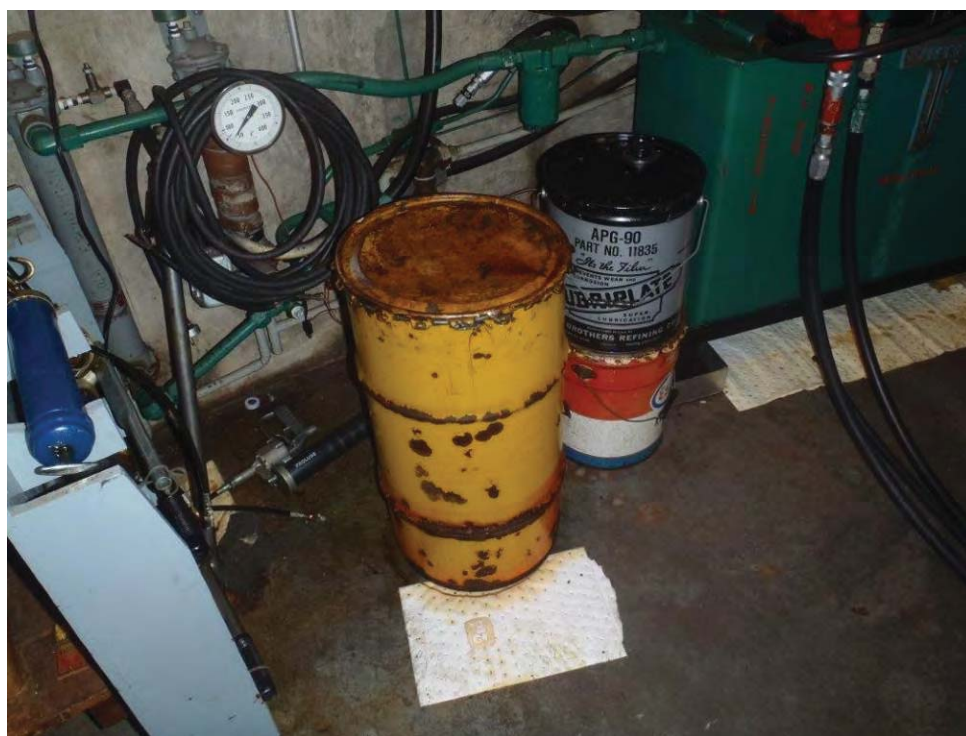
Photo 96: Drum leak at 43-meter Telescope.
