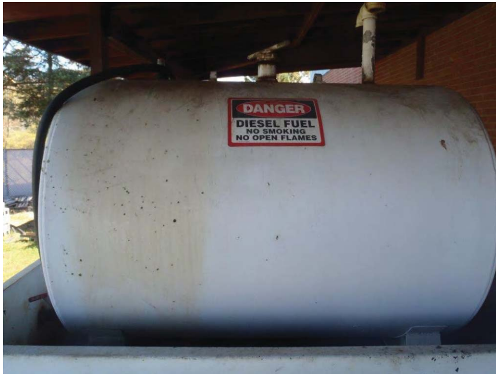
Photo 98: Diesel fuel AST behind Warehouse.
