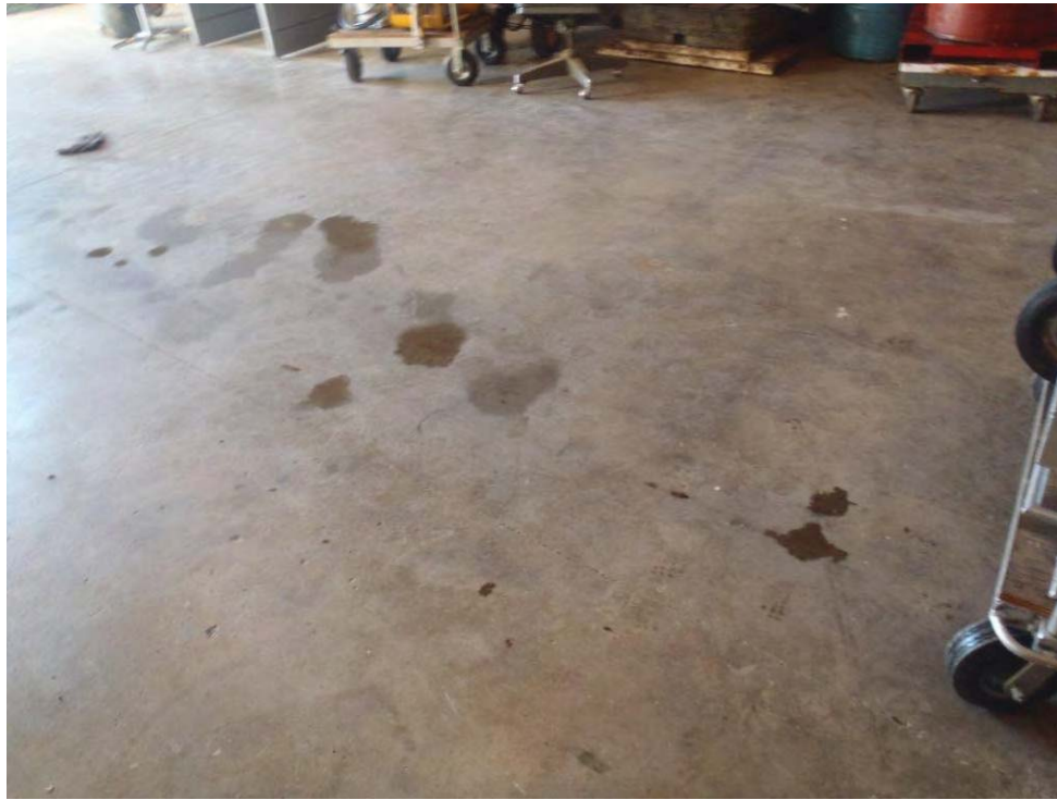
Photo 97: Staining of concrete floor inside GBT warehouse.
