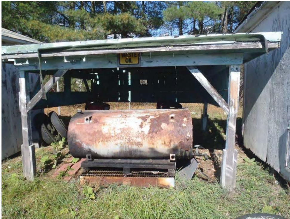
Photo 99: Waste oil AST at Work Area outside storage yard.
