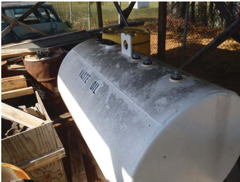
Photo 100: Waste oil AST at Work Area outside storage yard.
