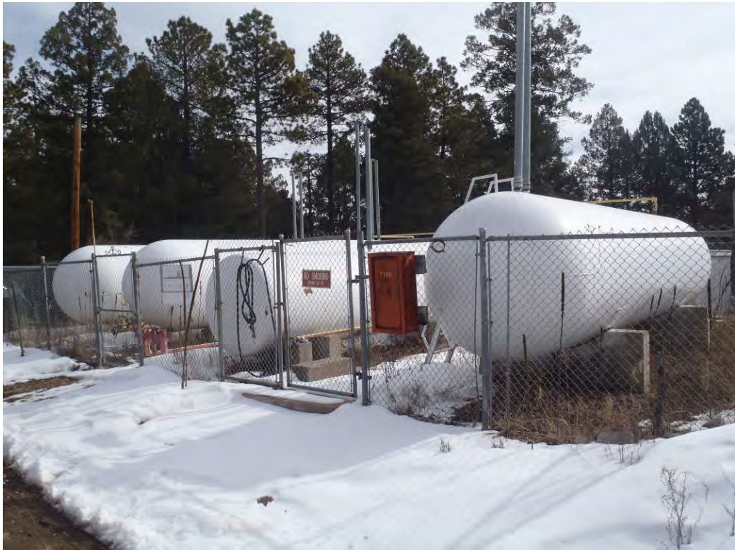
Photo 9: Propane tank yard facing northeast
