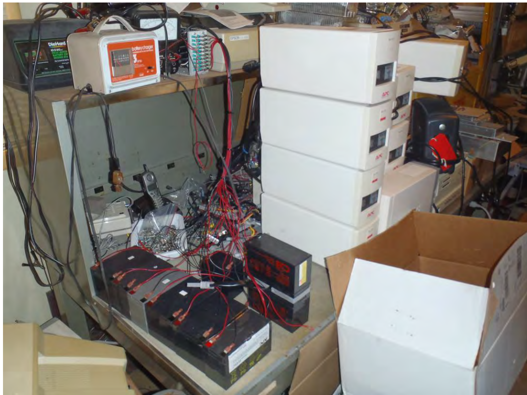
Photo 38: Battery charging area in main lab
