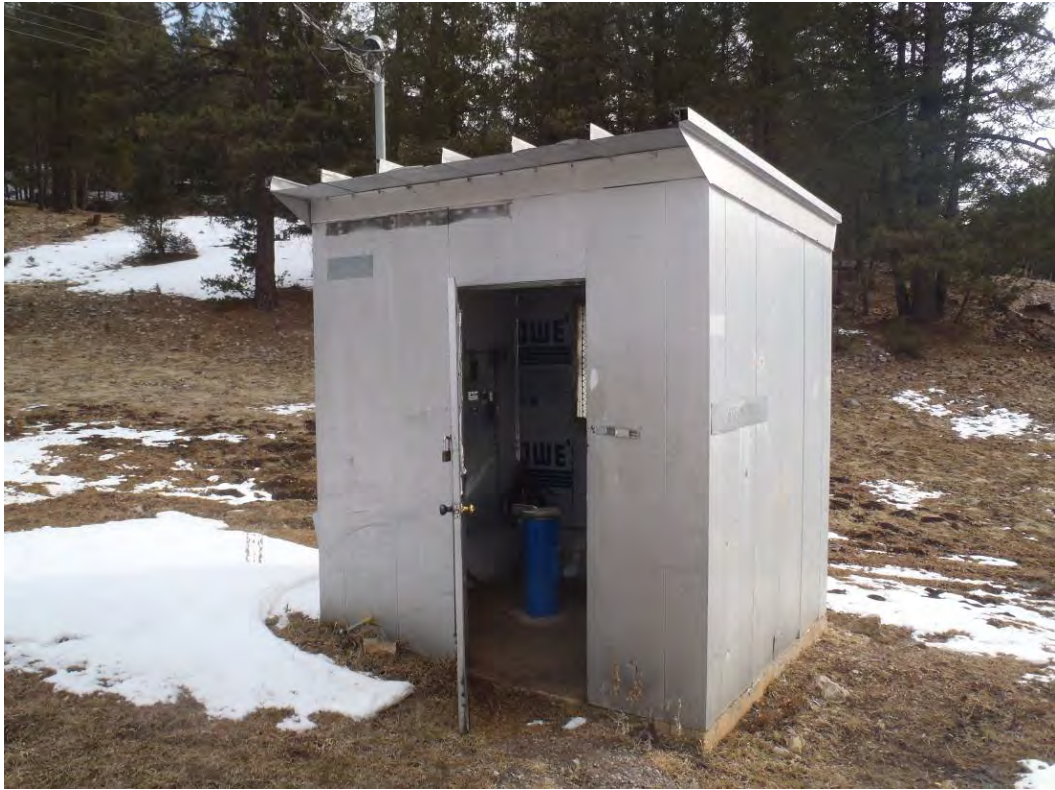
Photo 1: Water well #1 facing east
