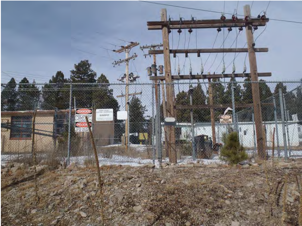
Photo 14: Transformers next to generator building facing west
