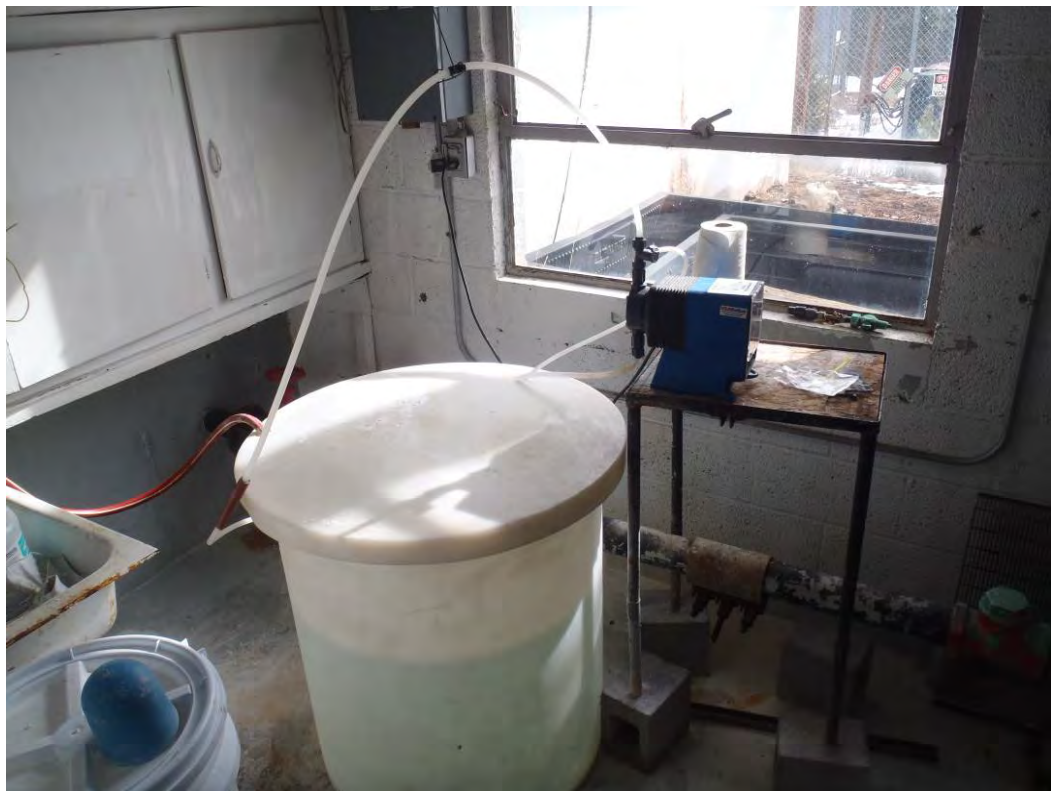
Photo 8: Supply water treatment chlorination tank
