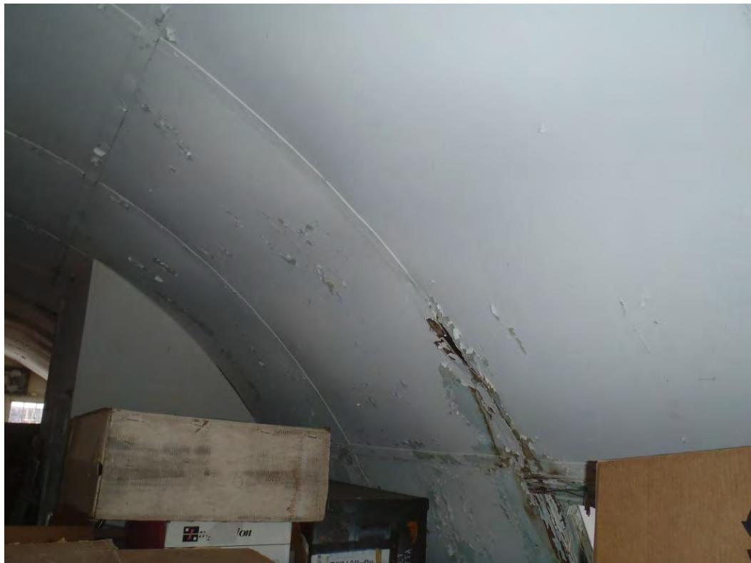
Photo 68: Paint peeling inside storage Quonset hut
