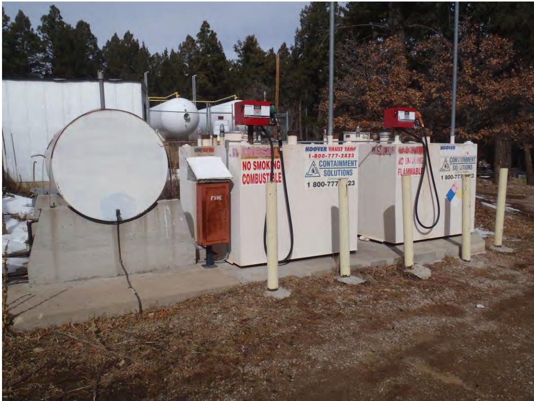
Photo 11: Fuel tanks facing west
