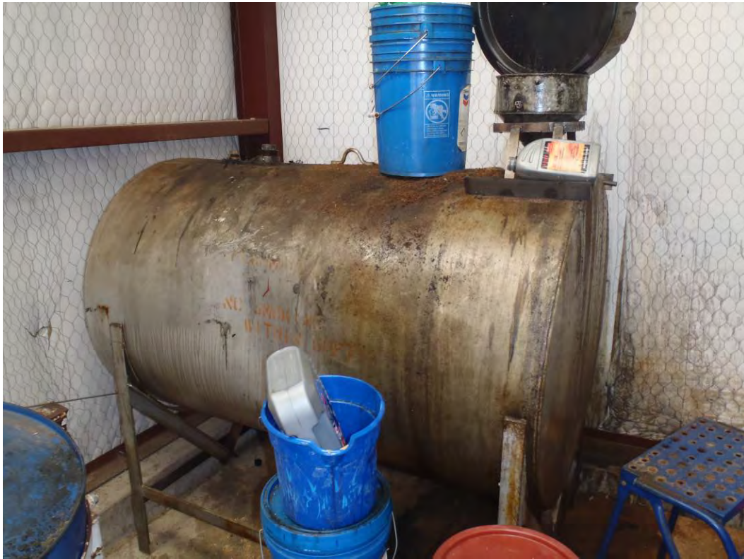
Photo 21: Used oil tank inside hazardous waste building
