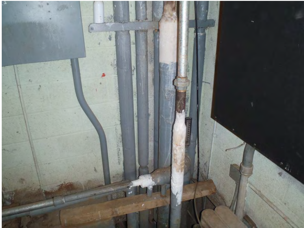
Photo 41: Suspected asbestos-containing material in main lab
