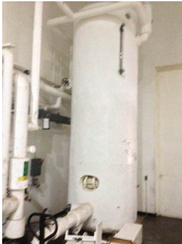
Photo 51: Glycol tank inside Dunn Solar Telescope
