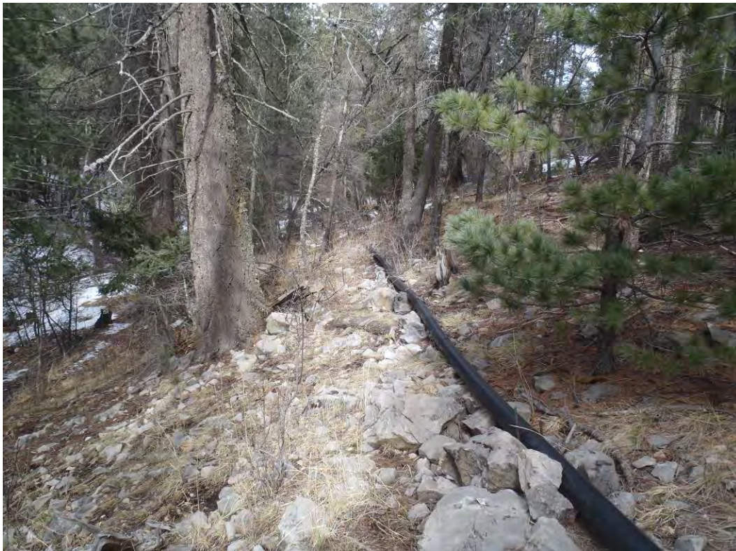
Photo 6: Wastewater discharge perforated piping facing northwest
