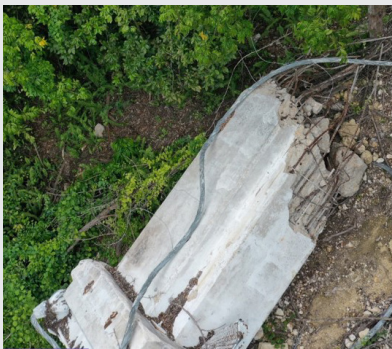
One of two fallen pieces of Tower 4 down the hill side
