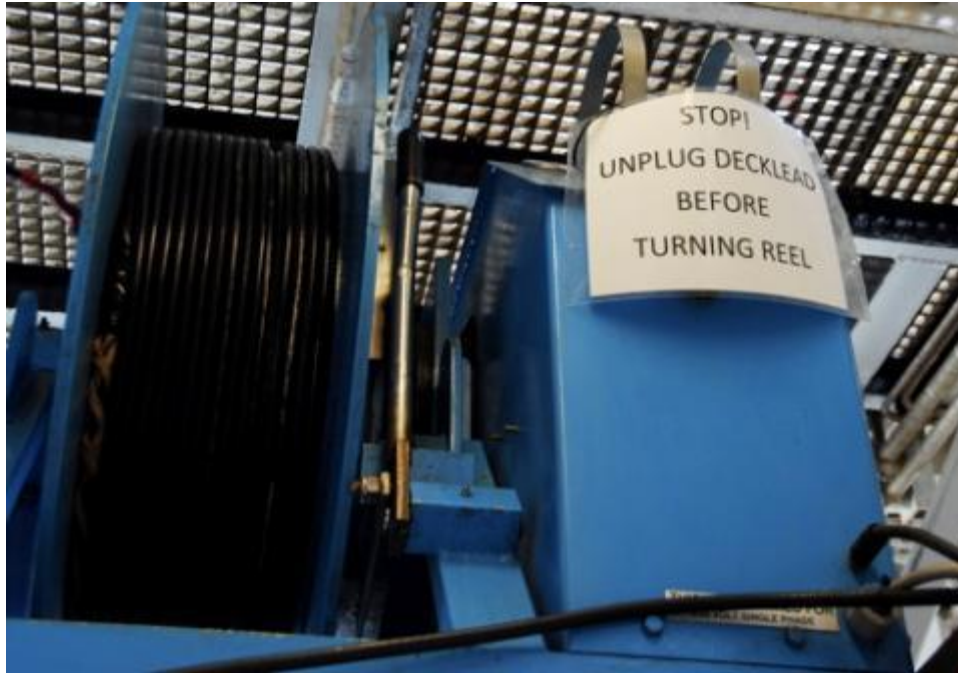
Figure 29. Deckhead winch on port stern gun deck with PAM hydrophone cable. Sign is placed over the switch that must be turned on to activate the winch. Winch cannot be operated while hydrophone cable and deck cable are connected
