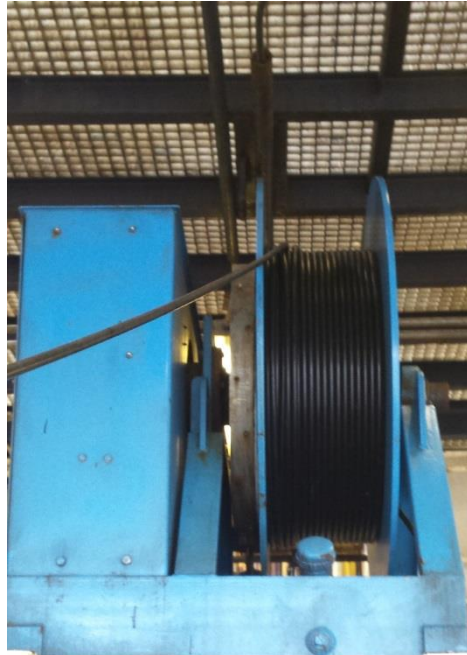
Figure 23: PAM tow cable spooled onto the winch and running aft.
