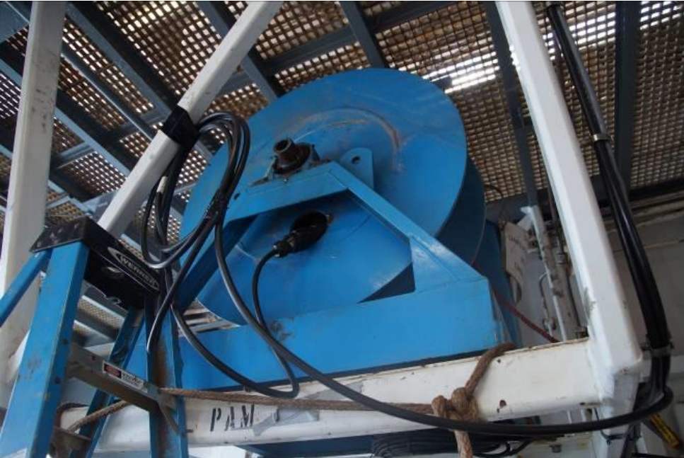
Figure 3: Hydrophone cable on the winch connected to the main deck cable.
