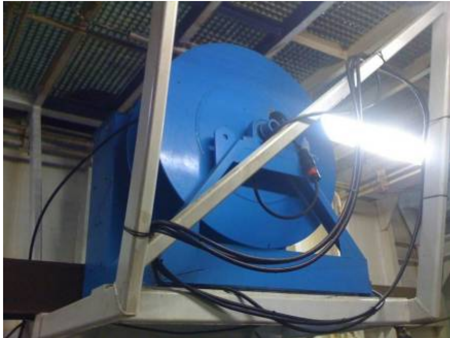
Figure D.3: Hydrophone cable on winch.
