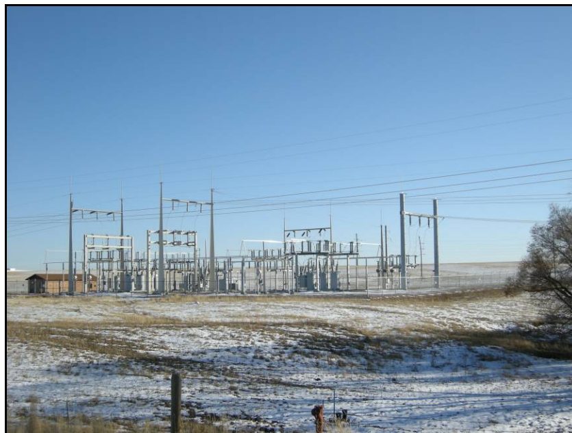
Figure 3-9. Happy Jack Power Substation (west of NRBP)
