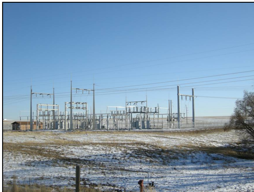
Figure 3-9. Happy Jack Power Substation (west of NRBP)
