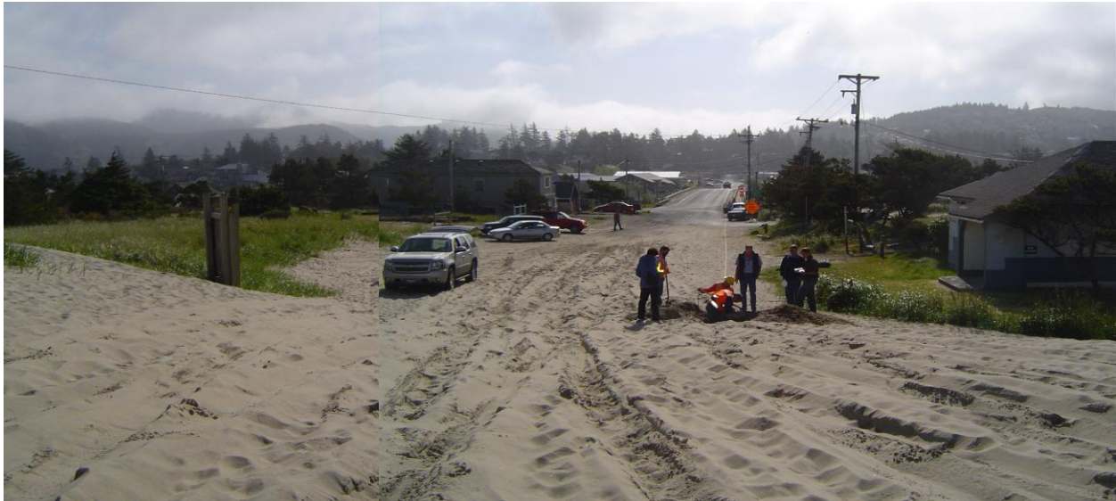
Figure 2-17. View to the East along Pacific Avenue Showing the Existing BMH at the Western End of the Parking Area
